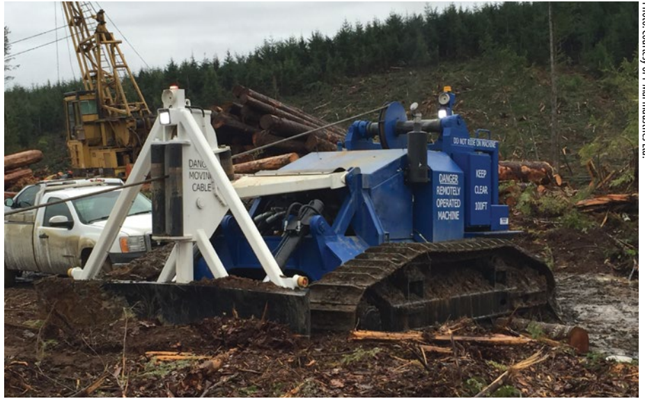
This remote controlled traction assist winch supports mechanized falling on steep slopes keeping workers off the ground and out of danger.
