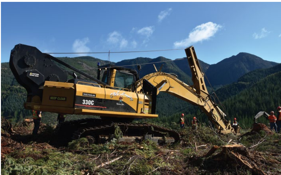
This excavator has EMS traction line winches attached to it and the operator in the feller buncher parked below is operating it by remote control.
