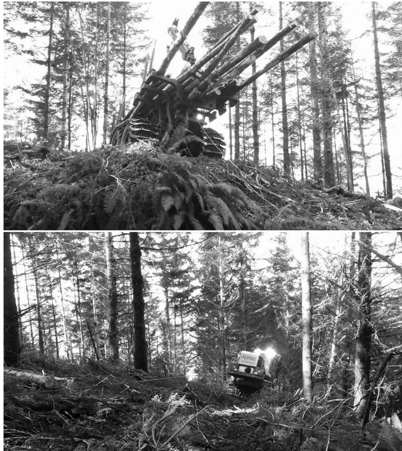
Figure 2. Ponsse Elephant King forwarder (above) and Ponsse Bear harvester (below) on tethered thinning operations in the Oregon Coast Range (photo taken by the lead author, Joshua Petitmermet).
